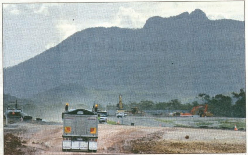
PROGRESS: View of trucks and the runway in front of Gladstone's iconic Mt Larcum. The completion date is expected to be at the end of May. Pictures: CHRISSY HARRIS airp140410-102
