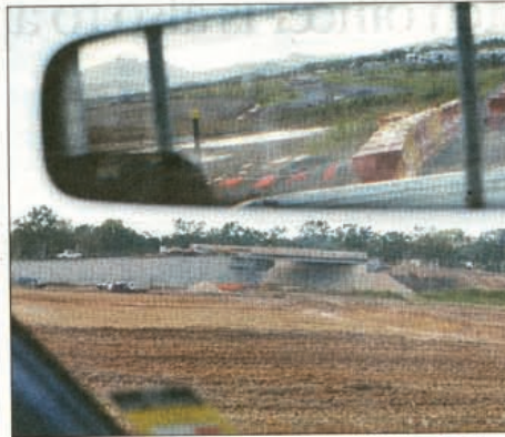
BRIDGE: The upgrade includes work on the bridge at the Callemondah-end of the airport.
