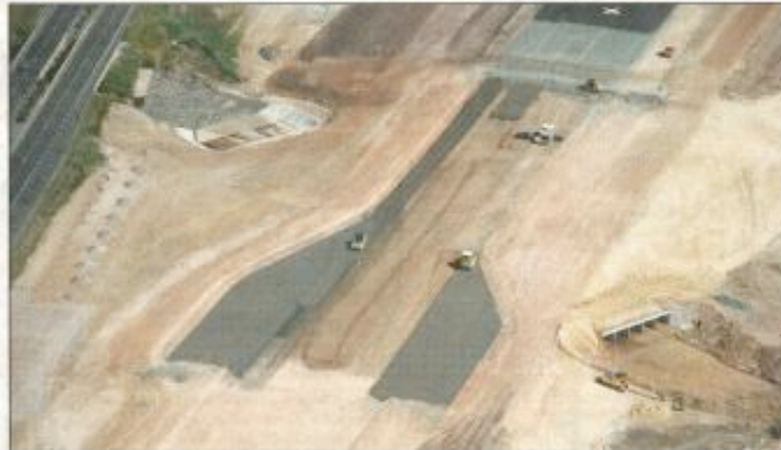
ZOOMING IN: The view of the Gladstone Airport expansion on May 5 about 1000ft up. Picture: MURRAY WARE
